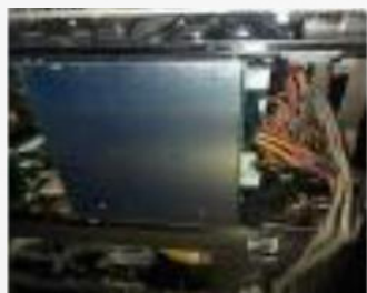
DC Power Box
