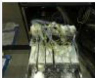
PR Pump Area
