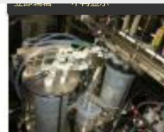
HMDS Buffer Tank
