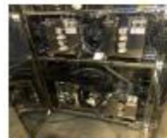
DEV Chemical Area
